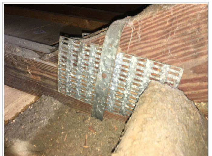
Metal Connectors not Meeting Nail Requirements
